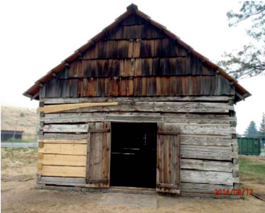
Figure 24. Front Entrance (West Elevation) of Skolaskin's Church upon Completion of Phase II Stabilization.
