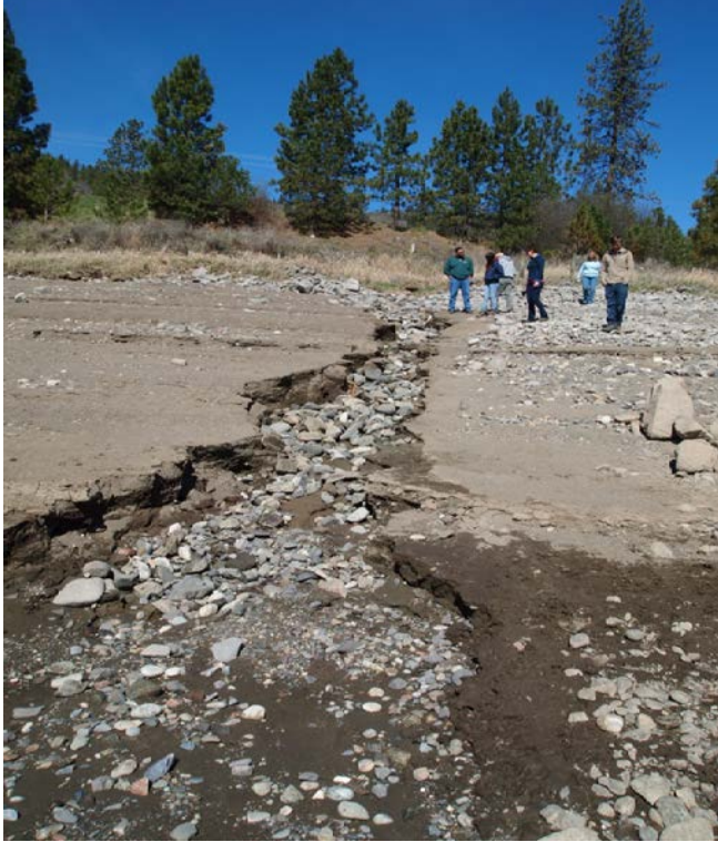
Figure 27. Spokane Arm Cooperating Group Inspecting Seasonal Erosion during a Spring Field Visit.
