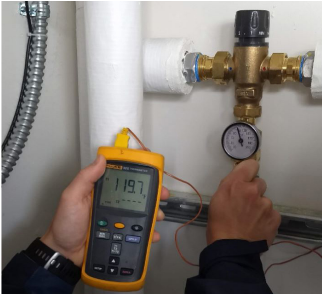
Figure 3. Thermostatic mixing valve with water temperature outlet of approximately 120°F.
