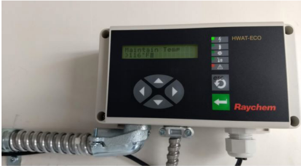
Figure 4. Temperature Maintenance heat trace set to maintain 116°F in distribution piping.
