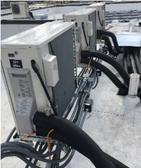
Figure 5. Rooftop Sanden HPWH with freeze protection heat trace.
