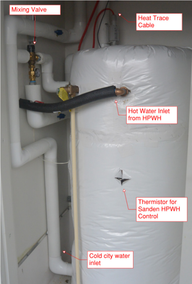
Figure 2. Hot Water Storage Tank on Level 4
