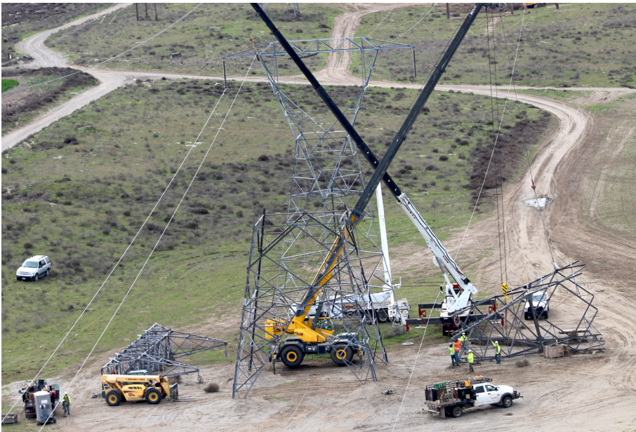
Transmission rates fund operations and maintenance work, like this Shepards Flat rebuild project, that helps ensure power is delivered reliably to customers.
