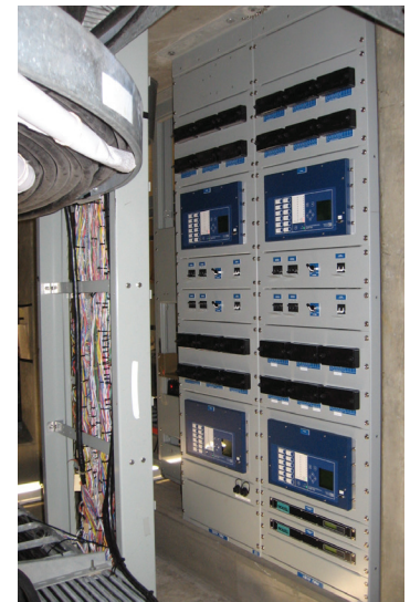
BPA has installed more than 100 phasor measurement units. These shoe-box sized devices transmit a feed of precise power system data that provides operators a higher-resolution view of the grid.
