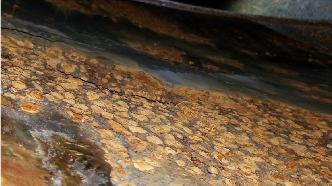
Picture 5: Typical Cavitation Damage – Pitting and Corrosion Close Up
