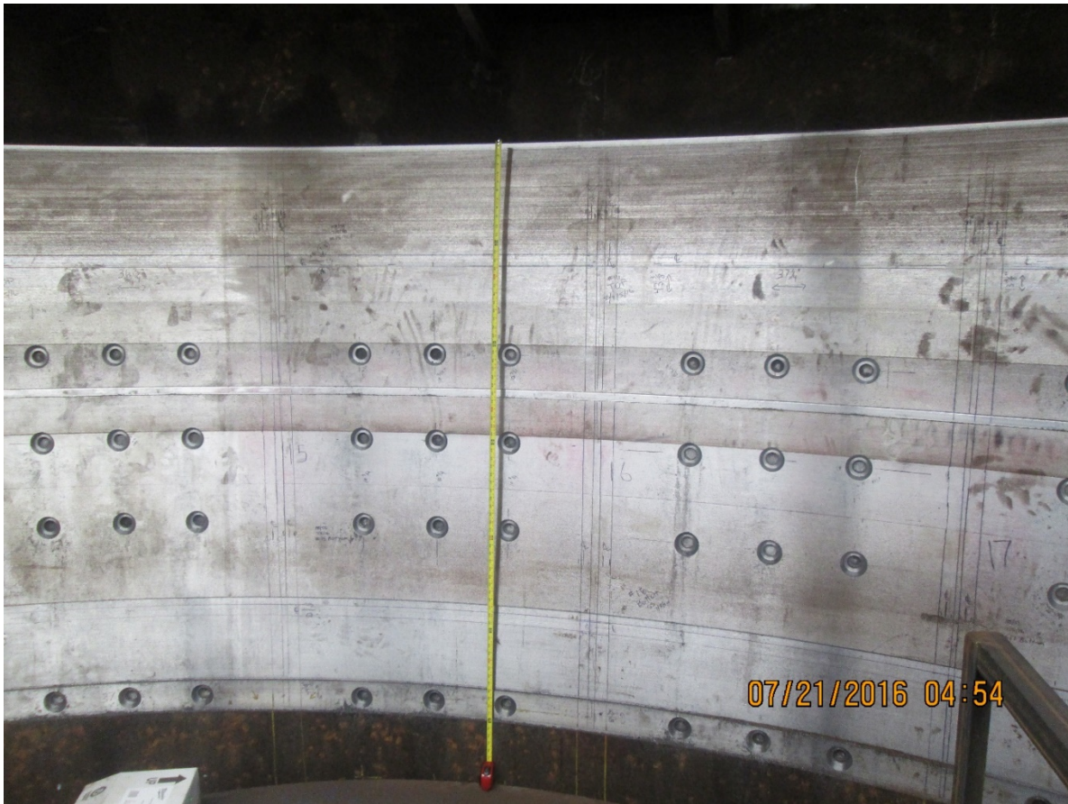
Picture 8: Discharge Ring Stainless Steel Liner Upgrade – Final Stage of Installation Replaces Portion of the Discharge Ring with a Stainless Steel Band Typical of Work Performed at Lower Monumental 2016
