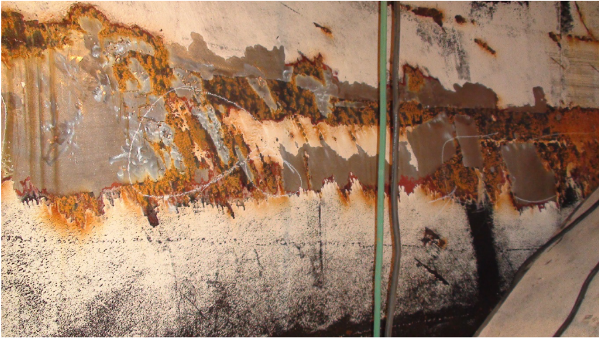
Picture 2: Typical Cavitation Damage on Discharge Ring and Previous Repairs: Observed New or Continued Cavitation near Repaired Areas.
