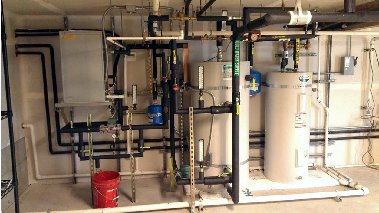
Figure 3: Phase 2 VRF Water Heating Plant Mechanical Room A
