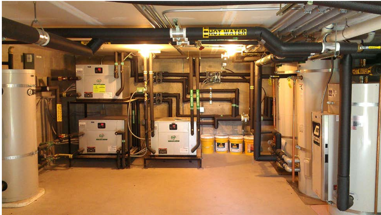
Figure 2: Phase 1 Geothermal Heat Plant Mechanical Room
