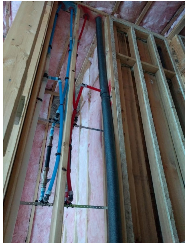
Figure 10. Heat trap installed in a building
