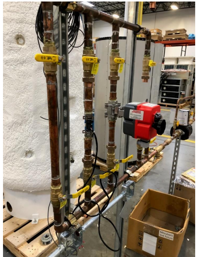
Figure 3. Heat exchanger and pump assembly control valve test setup
