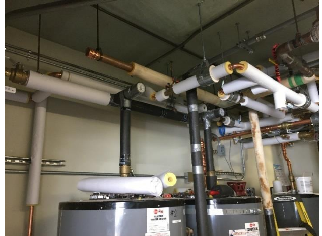
Figure 7. New piping in mechanical room connecting to existing electric resistance water heaters (during insulation installation).
