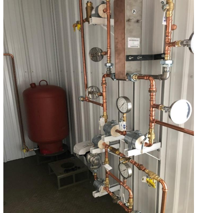
Figure 3. Secondary loop heat exchanger before pipe insulation was installed. Photo credit: Steffes.
