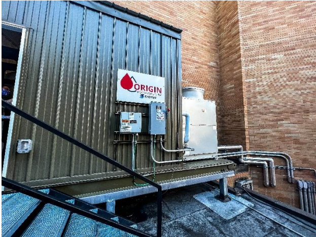
Figure 5. Origin skid installed at Bayview Tower with HEAT20 external to skid enclosure. Photo credit: Blue Fern Productions.
