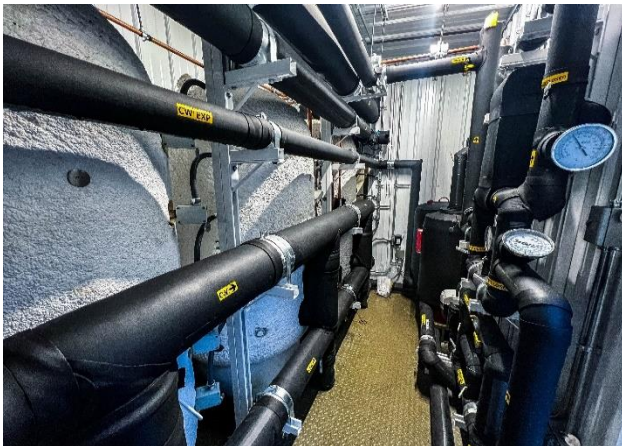
Figure 6. View inside rooftop skid shed with storage tanks (left) and secondary loop heat exchanger assembly (right). Photo credit: Blue Fern Productions.
