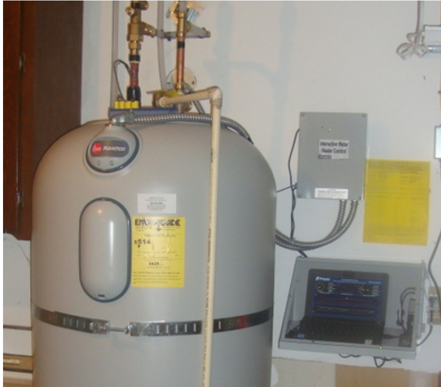
Figure 20: Installed 105 gallon water heater with Steffes mixing valve and interactive controls
