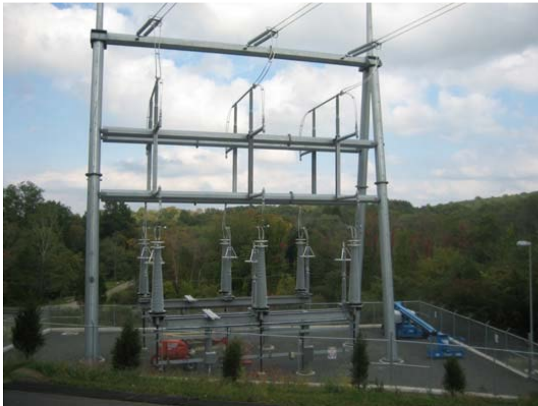
FIGURE 2-11 TRANSITION STATION AND STRUCTURES (WPSC PHOTO)
