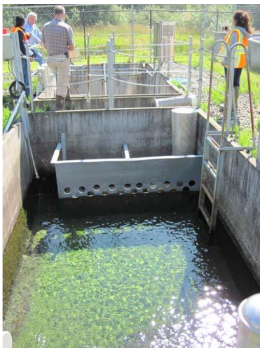
Photograph 2 – The settling basin and UV treatment system for the Burley Creek Hatchery (view looking east).
