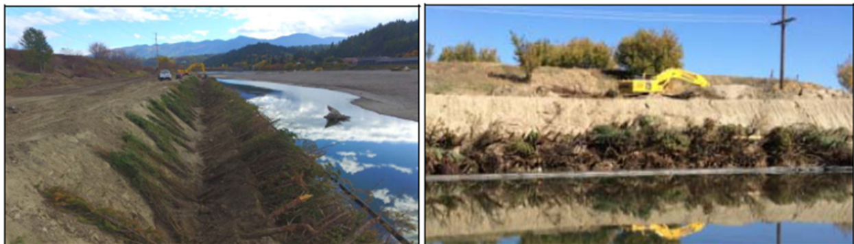
Figure 7 Vegetated brush bank structures under construction at the 2015 Bonners Ferry Islands project
