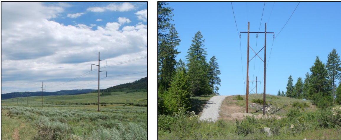
Figure 3-4. Typical Steel Pole (left) and Wood H-Frame (right) Transmission Structures
