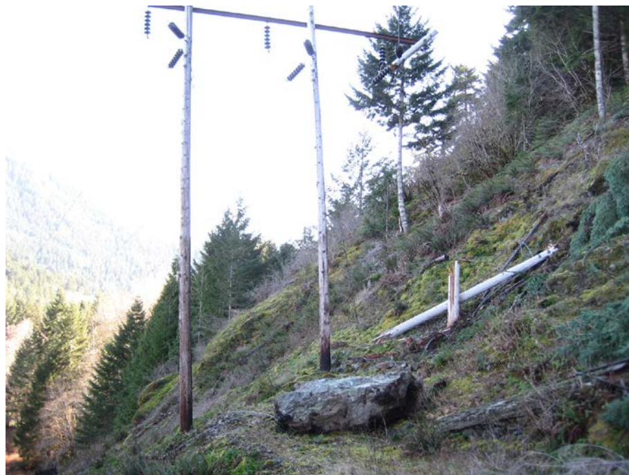
Figure 2-7. Damage to Existing Structure 2/7 (three-pole structure) from Rock Fall
