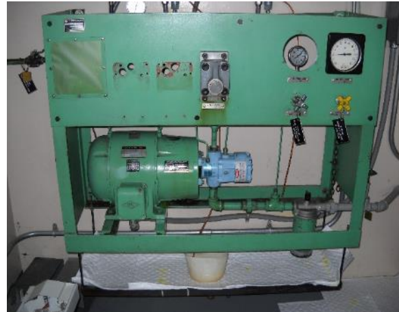
Photo 2: Pressurizing Unit Pump in Rigging Storage Room
