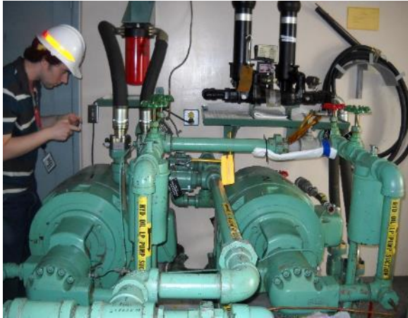
Photo 1: Power Unit Pumps in Rigging Storage Room
