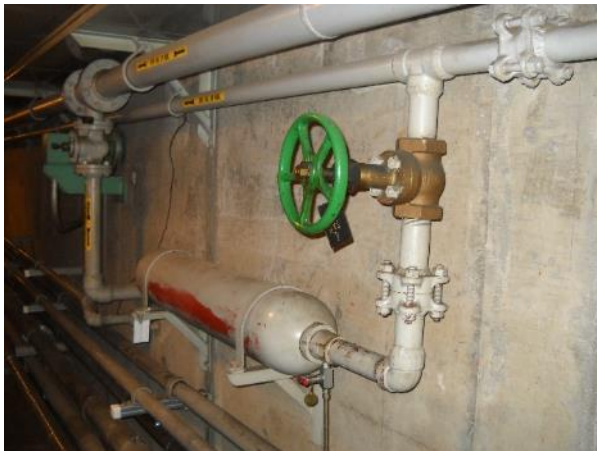
Photo 3: Piping and Accumulator in Pipe Gallery
