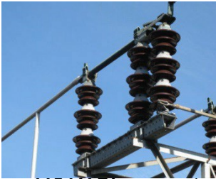
115 kV Disconnect Support
