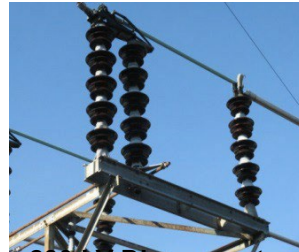
230 kV Disconnect Support
