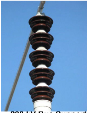
230 kV Bus Support
