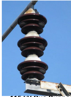
115 kV Bus Support
